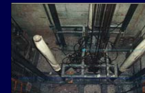
Elevator cable damage (another tall bldg., repaired in 3 weeks)
