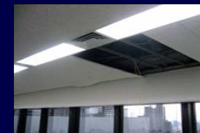
Falling of ceiling: 28F (21F, 14F, etc.)
